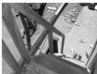
Some staircases are not age-friendly.
